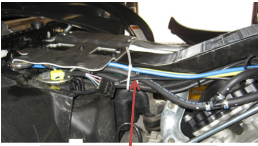
Note wires following manufacturers wiring route.
